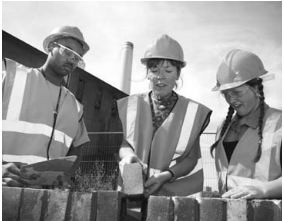
Philippa Langton (centre) joins students at Battersea laying the foundations of a new career
